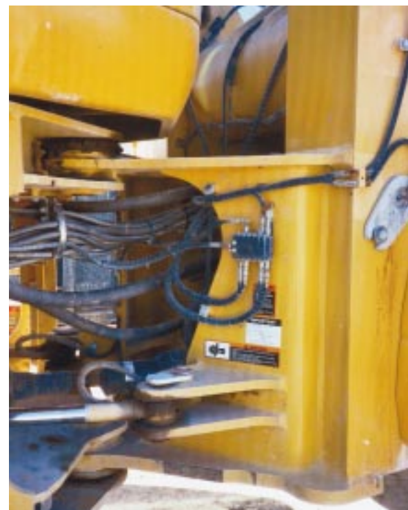
On this machine, the primary valve is mounted on the right-hand front frame. A 1/8-in. high-pressure hose is protected by spiral-wrapped guarding and spring coils.
