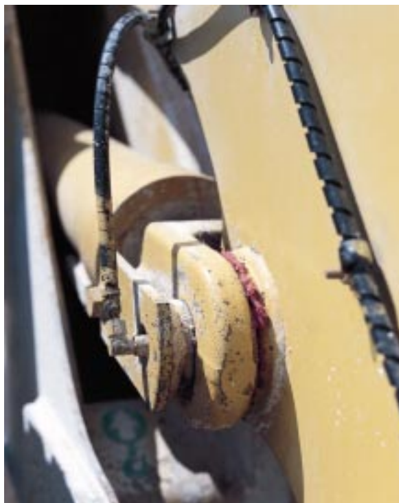
A perfect grease seal is visible on this wheel loader lift arm.
